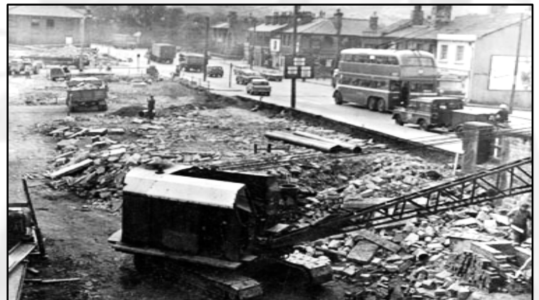
Demolition and road widening in Wakefield Rd. 1964. By courtesy of Kirklees Image Archive (k025014).
